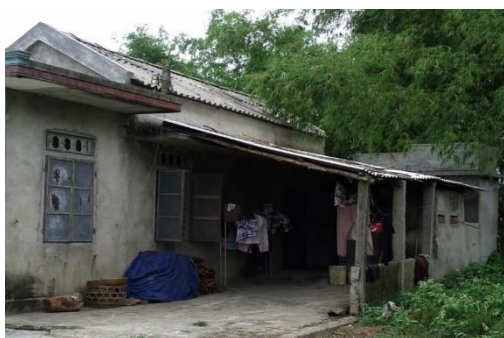
Fig. 9 Local residents' home with broken windows and molded concrete wall
