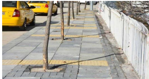
Figure 6: Failure guidance because of failure flooring, Pendik, İstanbul
