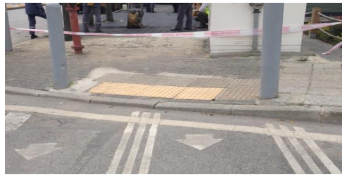
Figure 9: Failure yellow tactile pavings and failure ramp, Acıbadem, İstanbul
