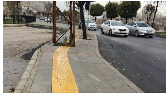
Figure 3: Electricity pylon on the yellow on the yellow tactile paving, İstanbul
