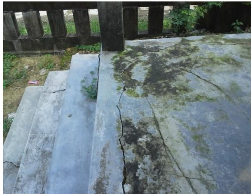
Fig. 23 Local resident's house with poor concrete slab at entrance
