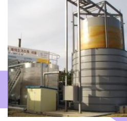
Food Waste Water Treatment Plant
